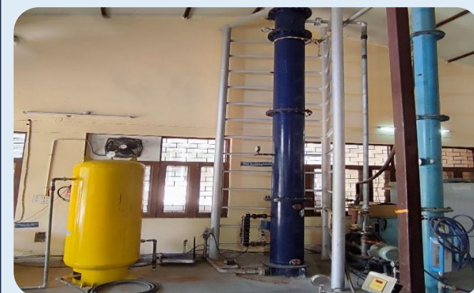
Biogas upgradation system at BDTC IIT Delhi
